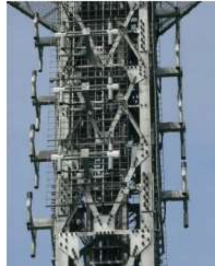
DMB Antenna System in Dae-ryong site
